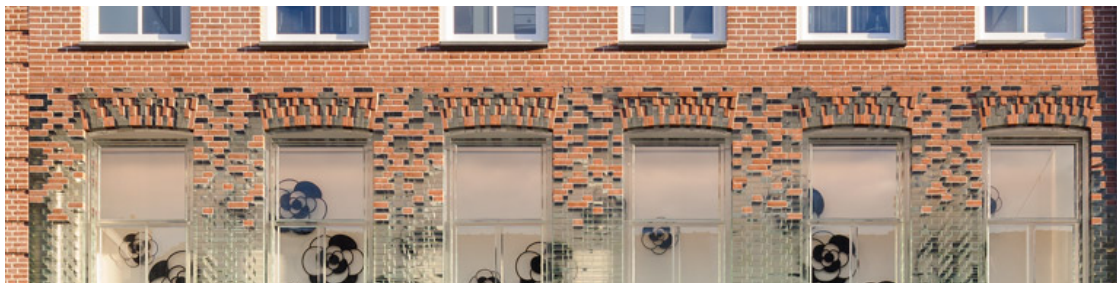
Figure 15. Brick Pattern on the Exterior of Amsterdam's Crystal Houses (Scagliola & Brakkee, n.d.)
