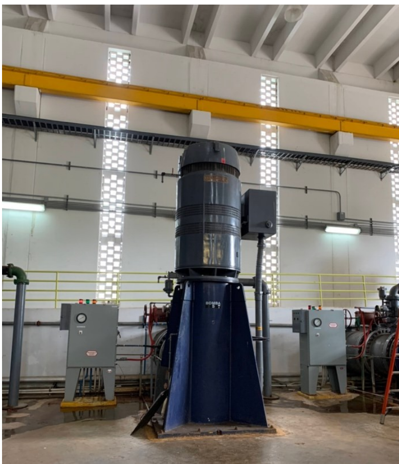
Figure 11. An intake pump inside the Lake Alajuela pump station (own photo)
