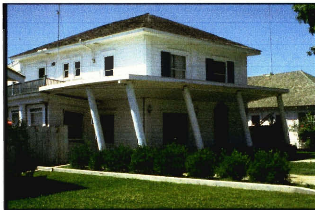
Figure 2.3: Soft Story Effects on a Structure Source: NGDC (2001b)
