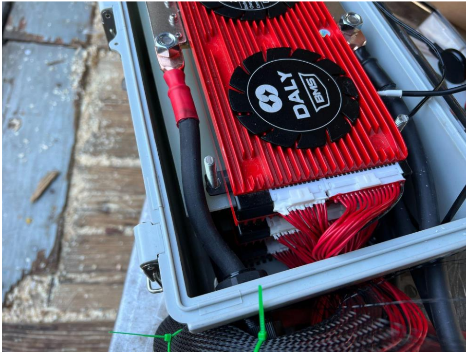
Figure 66. BMS Cable Management Inside Junction Box #2
