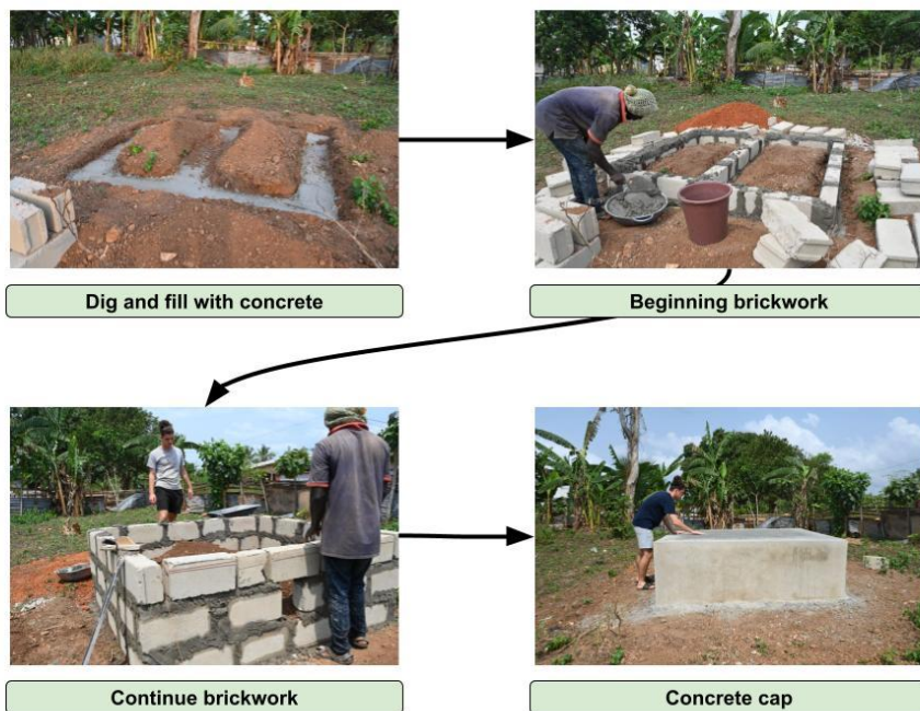
Figure 7: This is a diagram of the building process for the foundation. These are images of the foundation in different stages of assembly.
