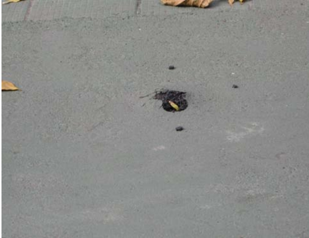
Picture K-13: Uneven Road Surface: Holes
