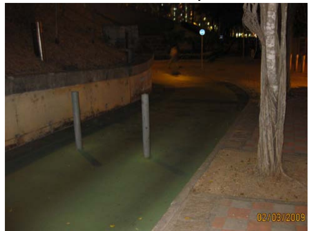
Picture K-10: Unnecessary Bollard
