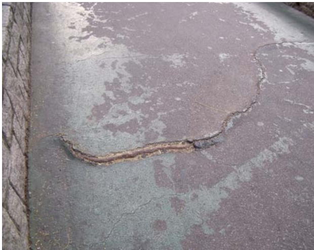
Picture K-11: Uneven Road Surface: Roots
