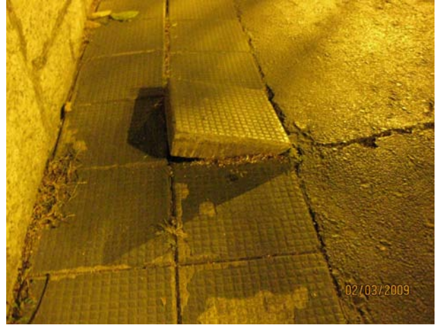
Picture K-14: Uneven Road Surface: Protruding Brick
