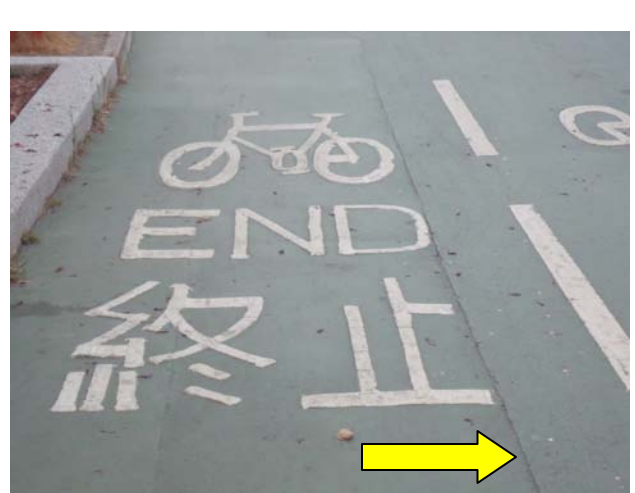
Picture K-12: Uneven Road Surface: Ridge
