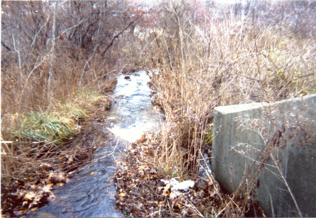
FIGURE 6: SEDIMENT BASIN FOUND ON INTERSTATE 190, CONTAINING SEDIMENT FROM THE HIGHWAY RUNOFF. ACCUMULATION OF THE SEDIMENT CAN CAUSE A PROBLEM. WATER MOVING AT A HIGH VELOCITY CAN ERODE THIS SEDIMENT MOVING IT INTO THE MILL BROOK.
