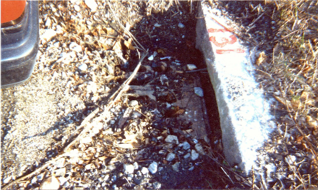
FIGURE 12: CATCH BASIN AT THE BASE OF WILDEY STREET. THE CATCH BASIN HAS SEDIMENT AROUND IT, SHOWING THE LIKELIHOOD OF SEDIMENT GOING INTO THE CATCH BASIN.
