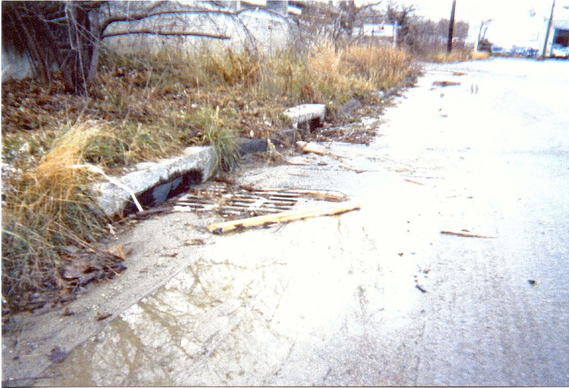
FIGURE 14: POORLY MAINTAINED CATCH BASIN ON PULLMAN STREET. THERE IS STREET SAND AND TRASH SURROUNDING THE CATCH BASIN.
