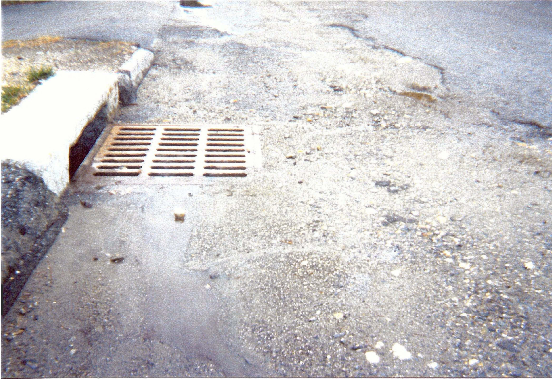
FIGURE 16: CATCH BASIN AT THE BASE OF TYSON ROAD. THE CATCH BASIN HAS SEDIMENT AROUND IT, SHOWING THE LIKELIHOOD OF SEDIMENT GOING INTO THE CATCH BASIN.
