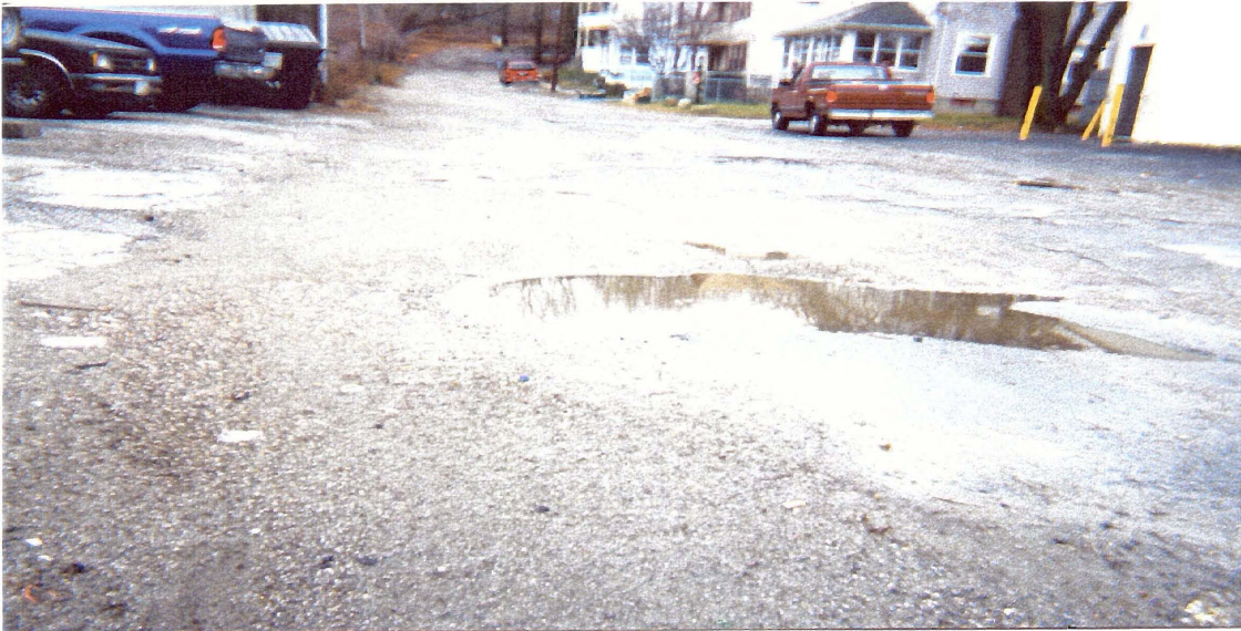
FIGURE 9: ASSUMPTION AVE AFTER A STORM. IT IS A PRIVATE UNPAVED ROAD. DUE TO THE STEEP INCLINE, WATER ERODES THE ASPHALT, CREATING TRENCHES THAT ARE FILLED WITH SAND AND GRAVEL. IN TIMES OF HEAVY PRECIPITATION, THIS SEDIMENT IS WASHED INTO THE CATCH BASINS AT THE BASE OF THE STREET.
