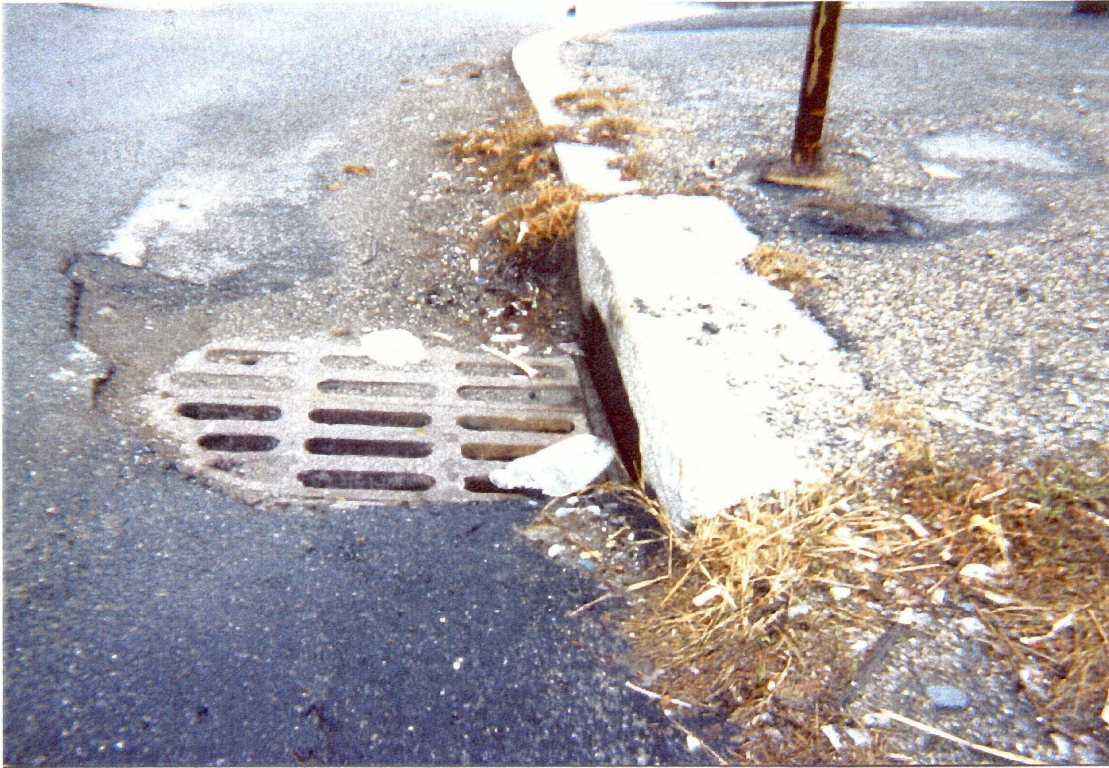
FIGURE 10: CATCH BASIN AT THE BASE OF ASSUMPTION AVENUE. THE CATCH BASIN HAS SEDIMENT AROUND IT, SHOWING THE LIKELIHOOD OF SEDIMENT GOING INTO THE CATCH BASIN.
