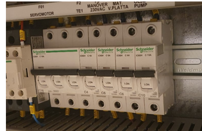
(b) Relay switches
