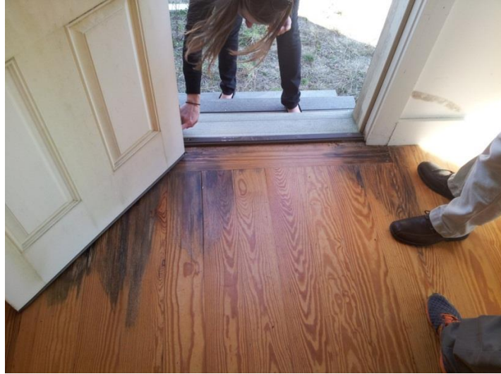
Figure : Water Damage Around Clifford House Door
