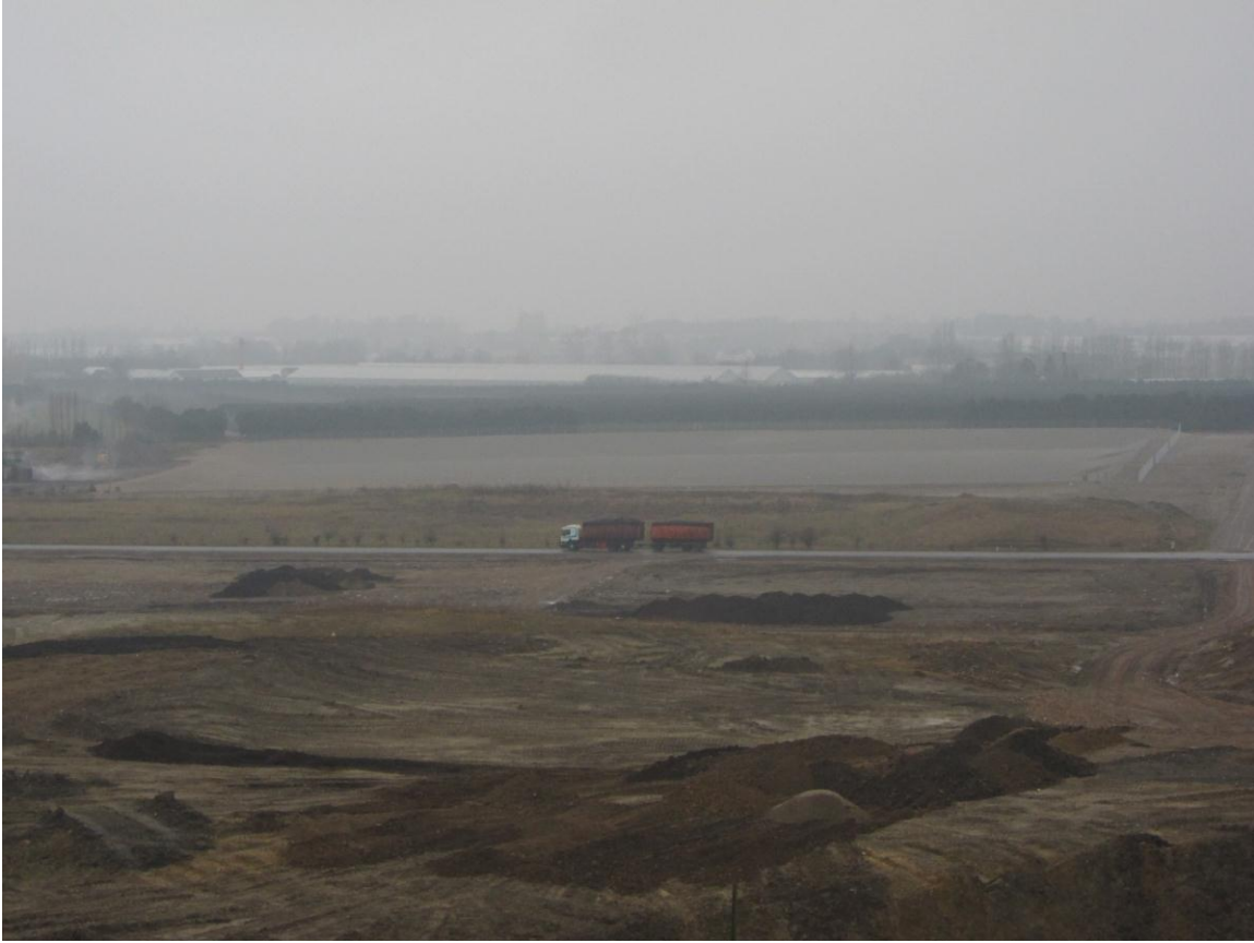
Figure 8: The bottom lining system of a new landfill cell can be seen off in the distance
