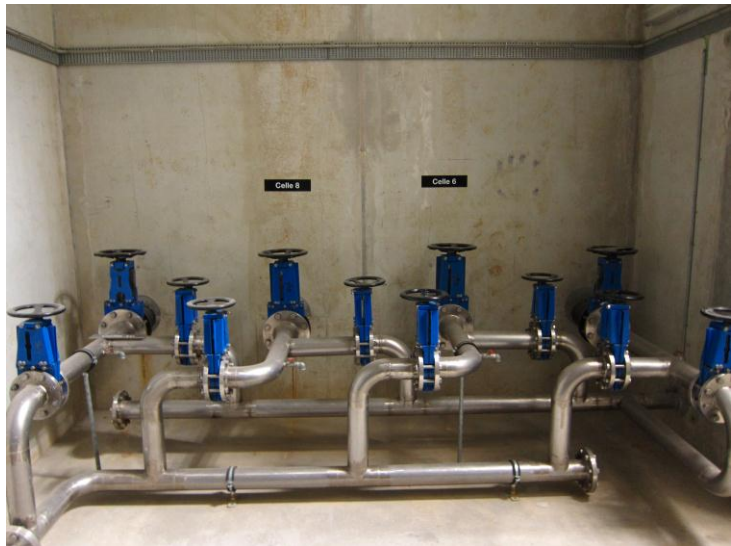
Figure 9: Leachate Collection System Valves
