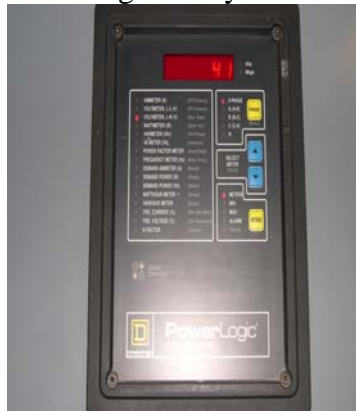
Figure 13: Advanced Digital meter for Alden and Riley Hall's
