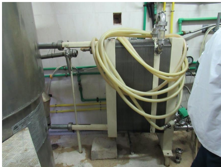
Figure 28: Closed loop heat exchanger at Birra Puka. Taken on Nov. 21, 2019.
