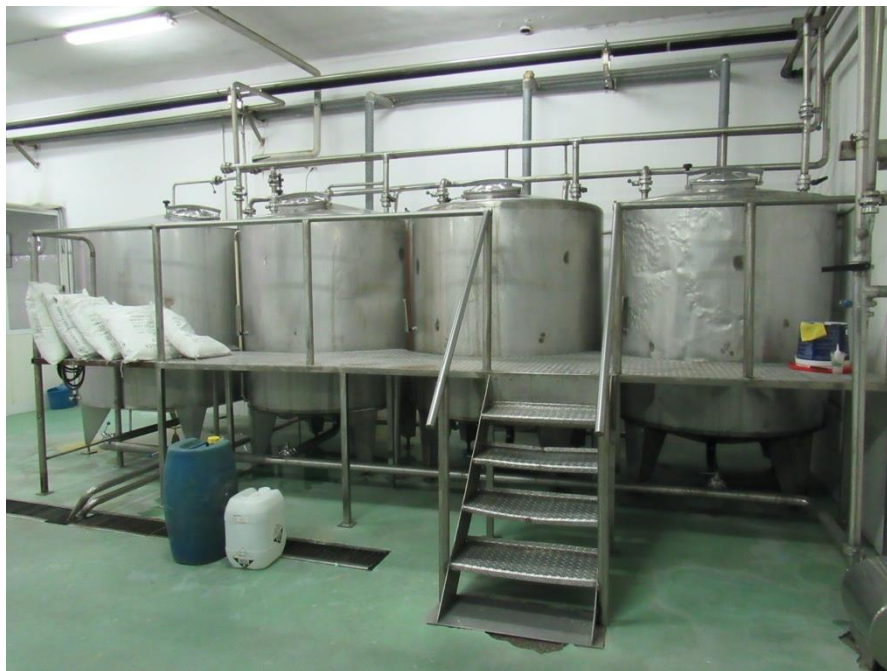
Figure 26: CIP system at Birra Tirana. Taken on Nov. 19, 2019.
