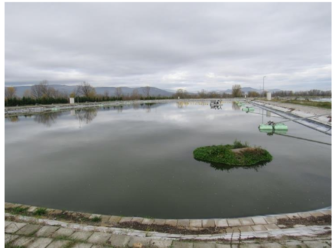
Figure 23: An aeration pond at Korçë WWTP. Taken on Nov. 15, 2019.
