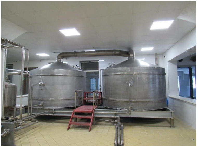
Figure 25: Wastewater neutralization tanks at Birra Tirana. Taken on Nov. 19, 2019.
