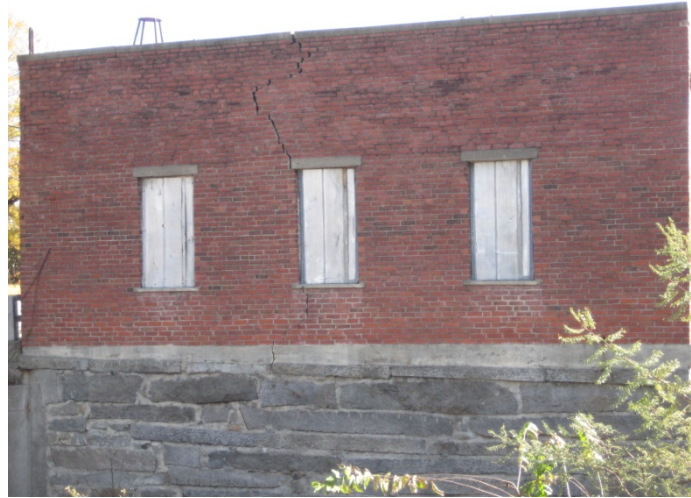
Figure 10: Exterior Structural Damage to Firehouse
