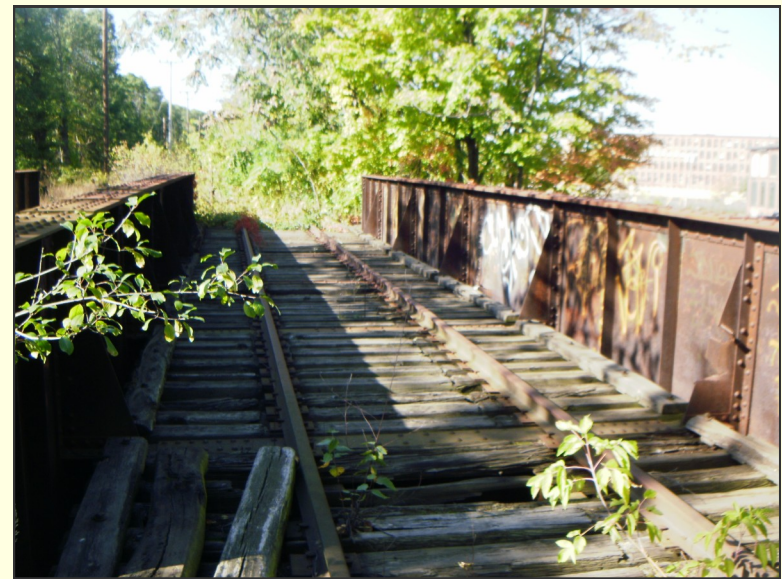
4. Figure 72: Gaps between ties on the Manchester Street Bridge
