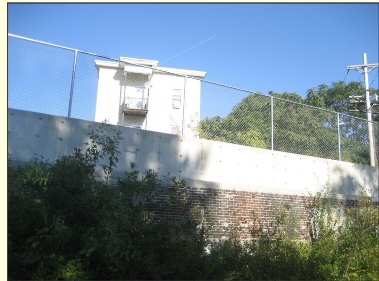
4. Figure 30: A brick and concrete wall along the northern part of the segment.
