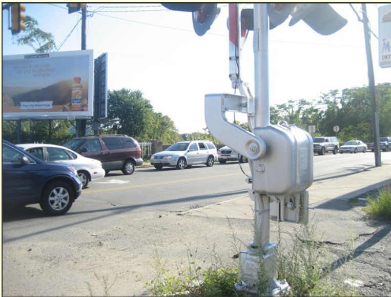
Figure 91: An existing railroad crossing system
