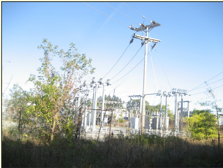
3. Figure 44: A power transmission facility
