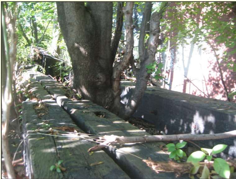
8. Figure 79: Large Wooden Structure that will need to be identified and removed
