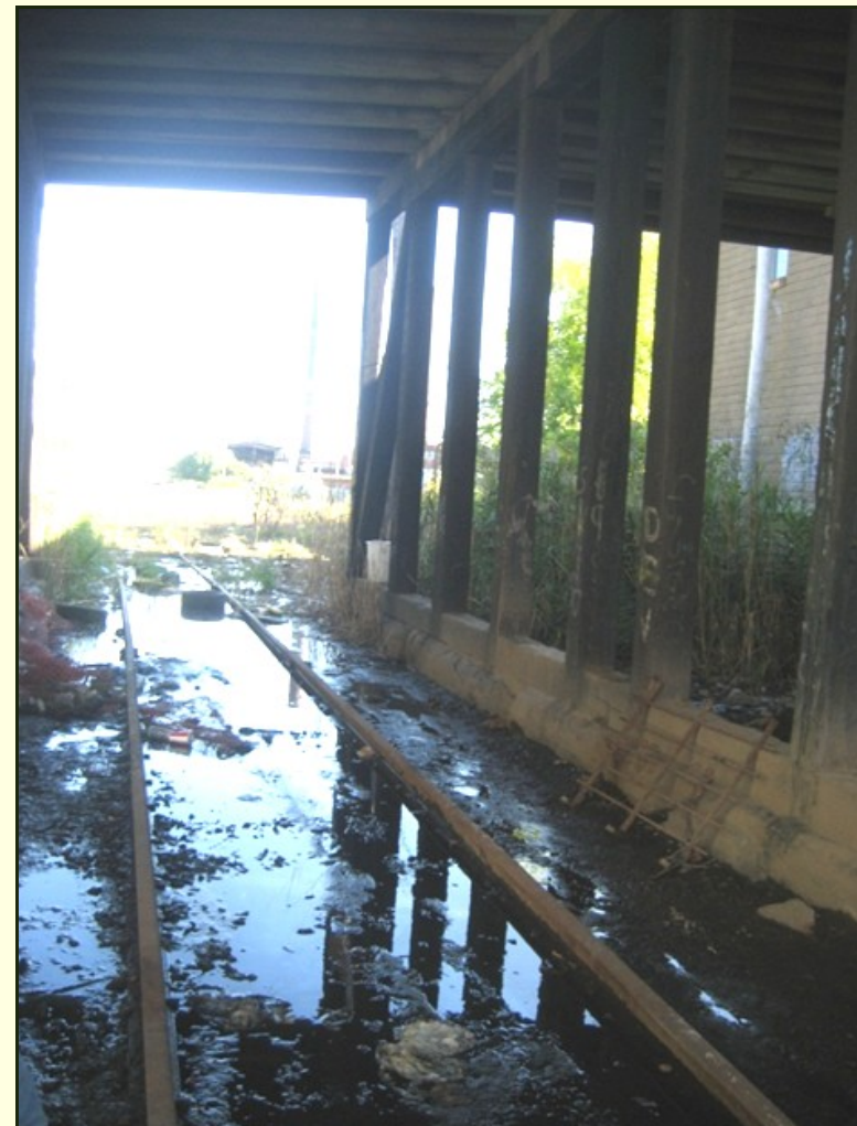
5. Figure 34: The drainage issues underneath the Lowell Street overpass
