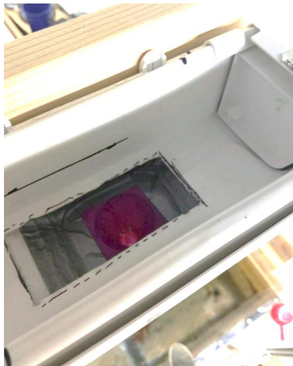
Figure 24: Funnels Placed on Top of Downspout
