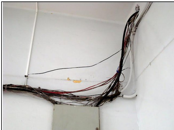
Figure 6: Exposed Wiring in Hospital San Juan de Dios
