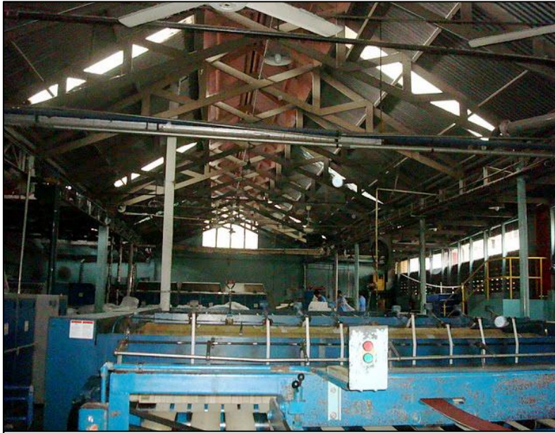
Figure 7: Ironing area in Hospital San Juan de Dios that had a lot of lint and dust on the ceilings and floors
