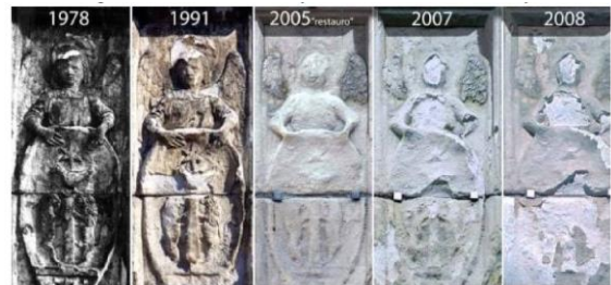
Figure 5 - Thirty Years of Deterioration
