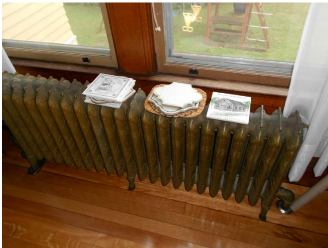
(Figure 4) Radiator on the first floor in Worcester Friends Meetinghouse
