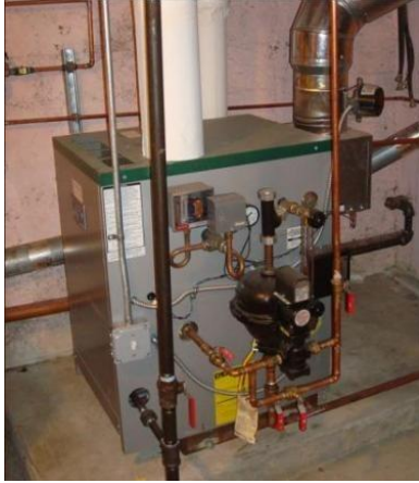
(Figure 1) Steam boiler
