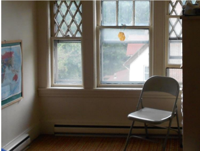
(Figure 3) Electric resistance heaters in the classroom on the third floor
