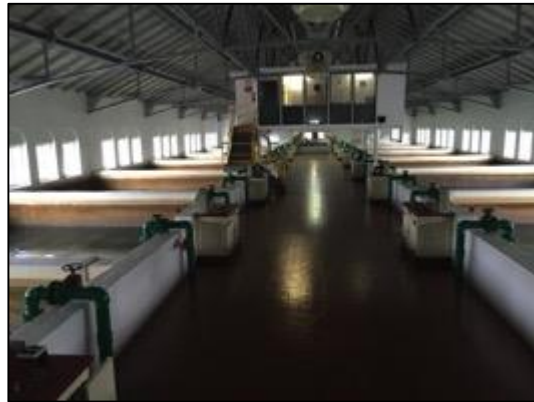
Figure 48: Water Filtration Chambers
