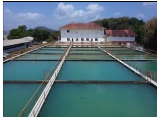
Figure 44: Water Treatment Basins
