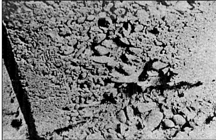
Figure 90: Cavitation in concrete (ACI Committee 210, 1998)
