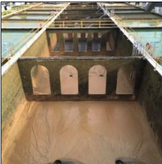
Figure 47: Sedimentation Sludge at Bottom of Basin
