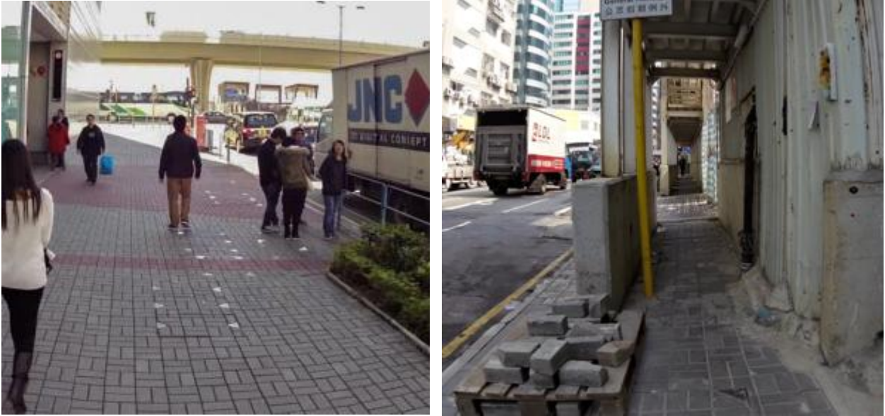
Figure 4.3: Sidewalk Condition Comparison of Lai Yip Street (left) and Tsun Yip Street (right)
