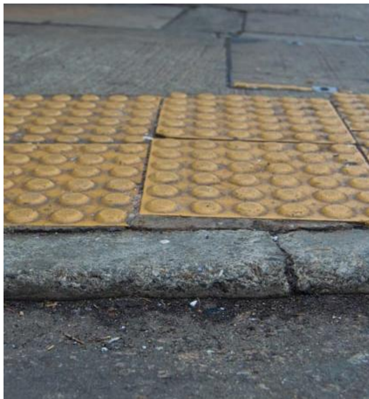
Figure J.1: Image of Lack of Cub Ramp
