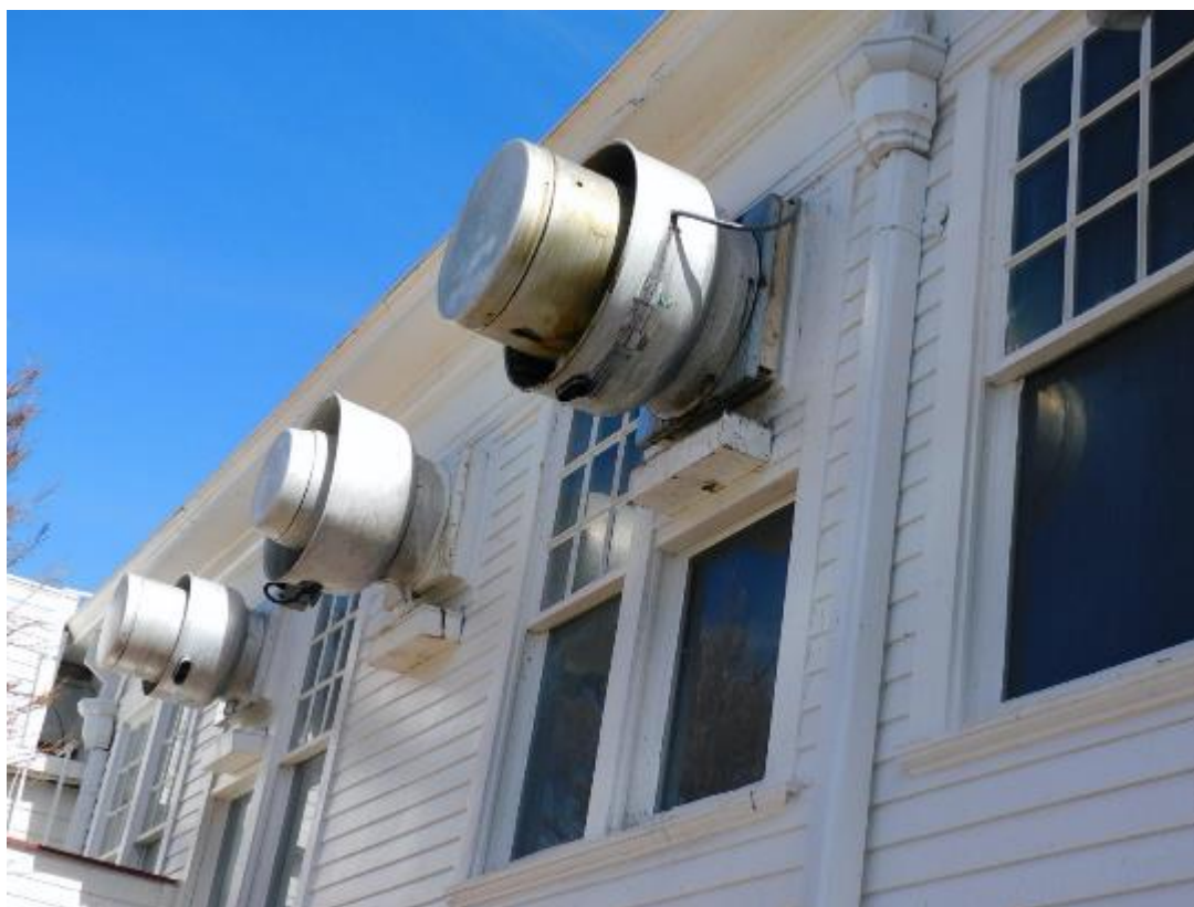
Figure 29. Image of air vents at a local business where grease was dripping from and creating a trail below.
