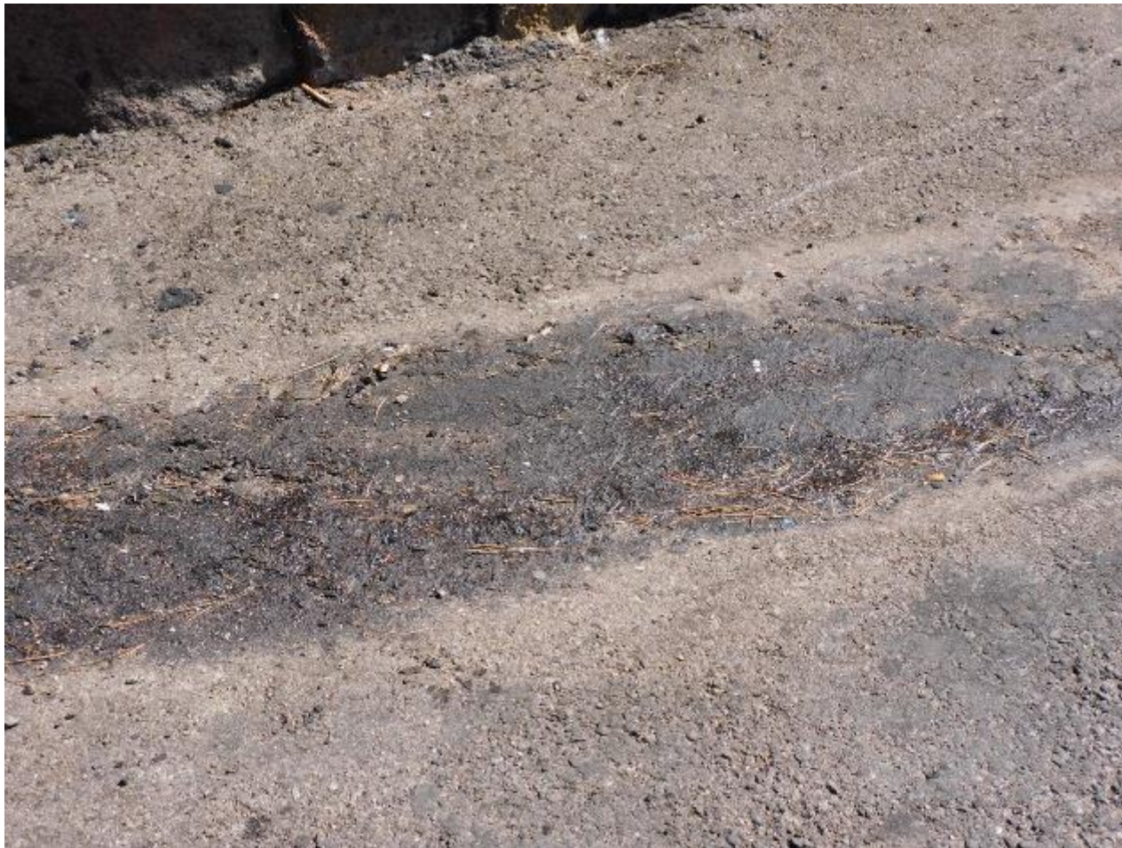
Figure 30. Image of grease trail created from the air vents in Figure 27.
