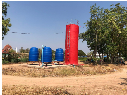
Figure 18. Water tanks in Nong Wang, red tank was installed by PDA and the blue tanks were not in use
