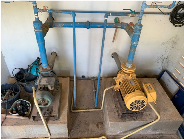
Figure 5: Surface pump in Nong Wang
