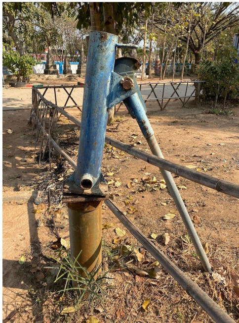
Figure 4: Photograph of a manual pump in Khon Kaen
