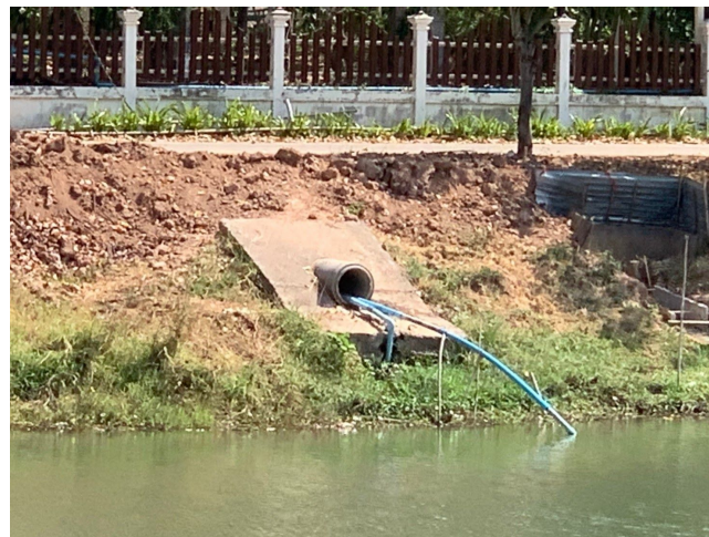
Figure 17. Water from the Chi River pumped into the man-made pond by a grid-powered water pumping system.
