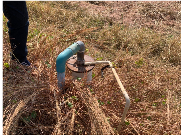
Figure 6: Submersible pump in Ban Lan
