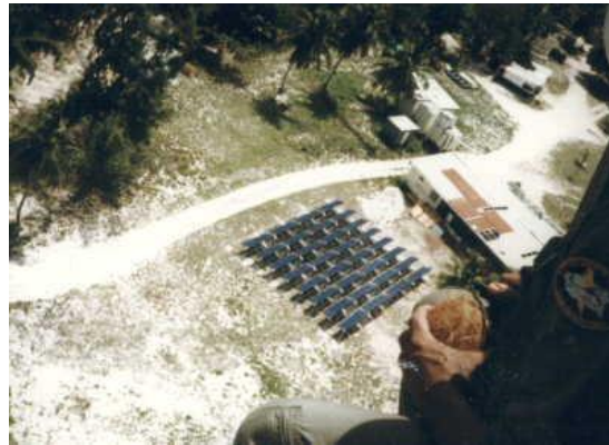
Figure 2.7: 15 kW Photovoltaic System on Mona Island, Puerto Rico (Bing, 1998)
