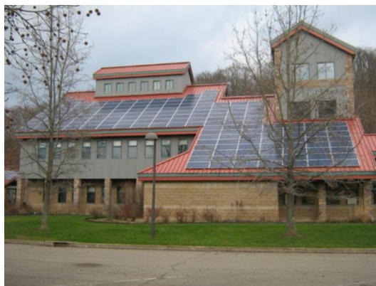
Figure 2.6: 59 kW Photovoltaic System at Wayne National Forest Headquarters (Sound, 2010)
