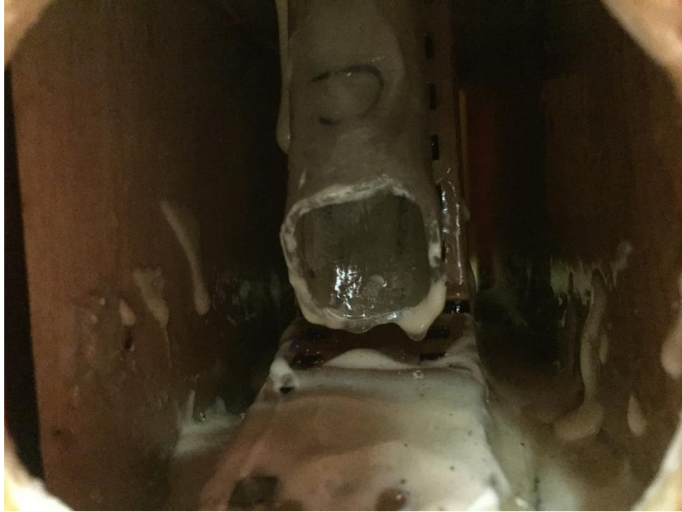
Figure 7: Epoxy on the interior side of the keel insert cavity.
