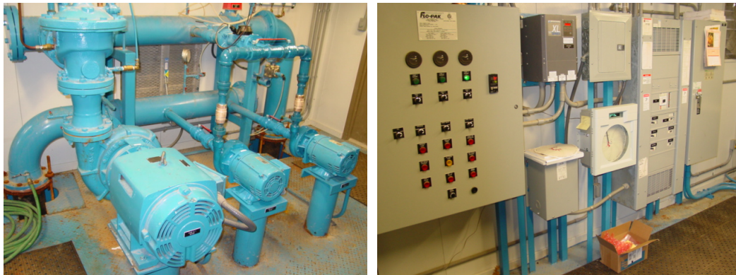
Figure 8: Booster Pumps and Controls
