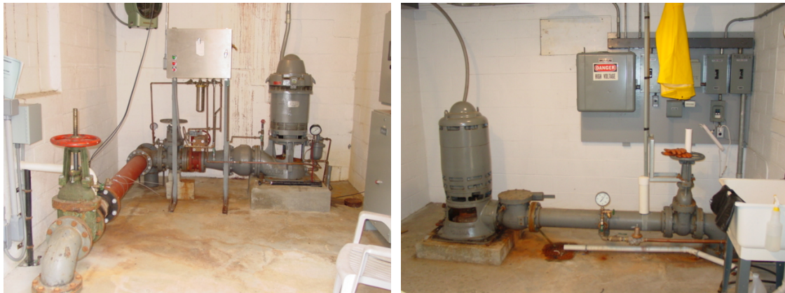
Figure 9: Well pumping Station and Components
