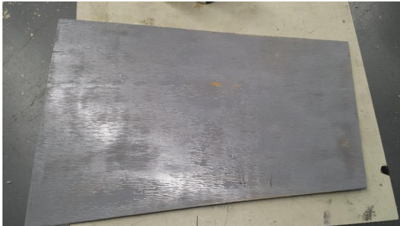
Figure 12: 1 completed side of diverging section-- Plywood sheet sanded and coated in primer and glaze
