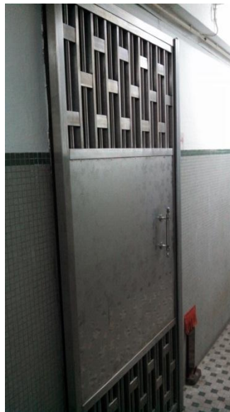
FIGURE 21: AN EXAMPLE OF A CAGE DOOR LEADING TO A BLOCK OF SUBDIVIDED UNITS.
