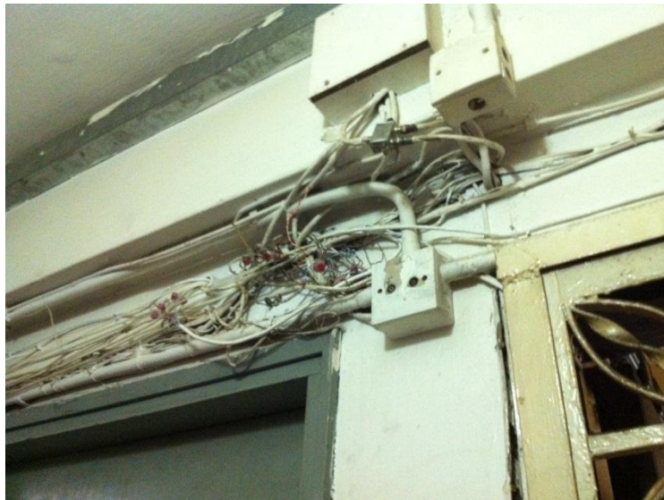
FIGURE 20: AN EXAMPLE OF DANGEROUS ELECTRICAL WIRING NOTICED BY OUR TEAM IN A SUBDIVIDED BUILDING.
