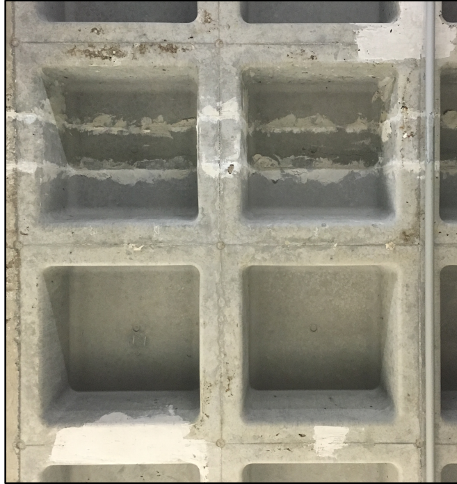
Figure 2: Underside of Waffle Slab on the Ground Floor of the Gordon Library
