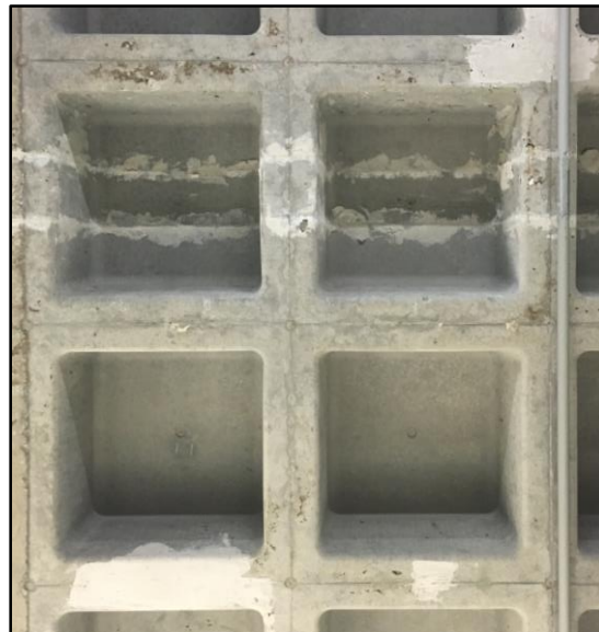
Figure 2: Underside of Waffle Slab on the Ground Floor of the Gordon Library
