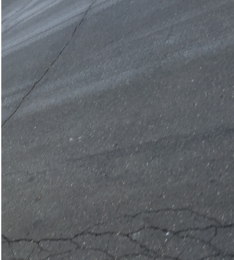
Figure 4.1: A picture of a road. This image includes variances in the road, such as cracks and wear. These are expected to be encountered on drivable roads, and a road detection test should account for them.
