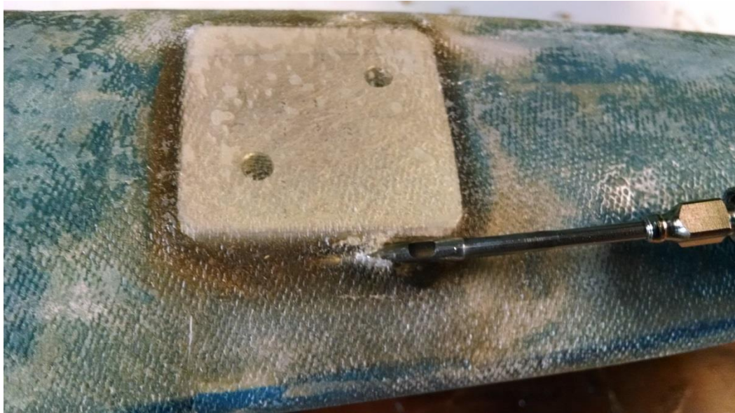
Figure 38 - Basting needle injecting epoxy resin into gap between fiberglass, plate, and hull
