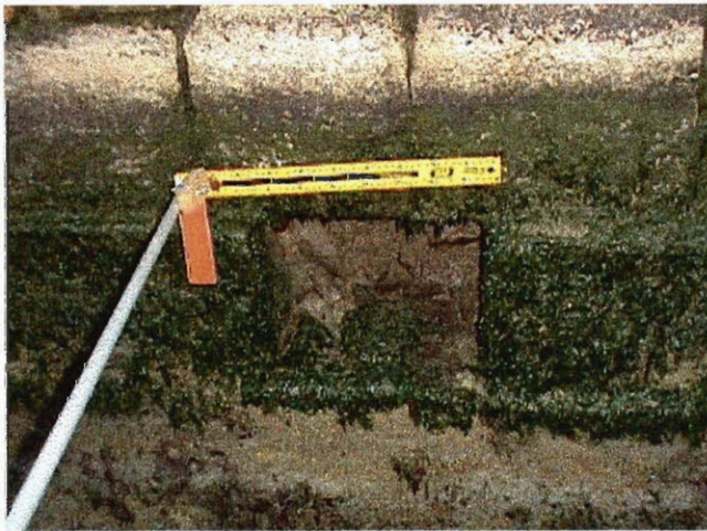
Figure 5-2 Sewer outlet with seaweed inside, a sign that it is inactive
