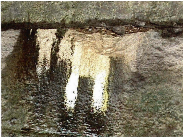
Figure 5-4 Beginning of a structural damage caused by leaking sewage pipes
