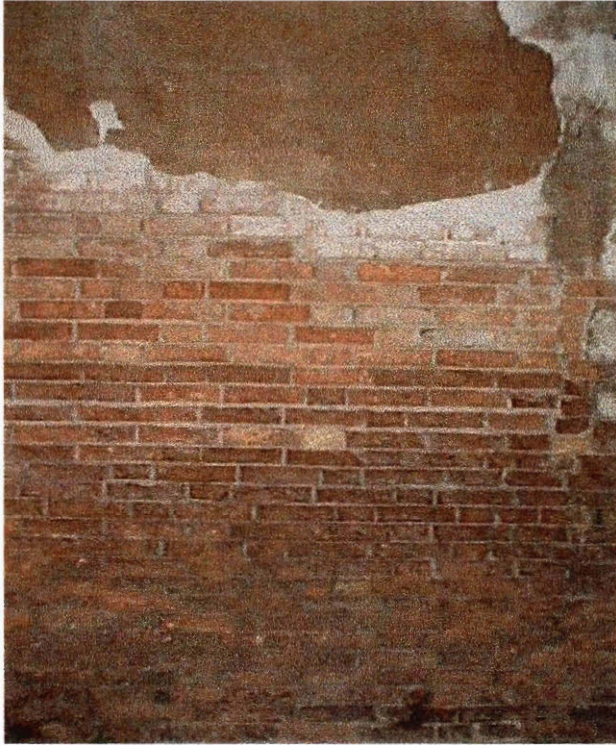
Figure 5-1 Wall segment showing partial plaster erosion
