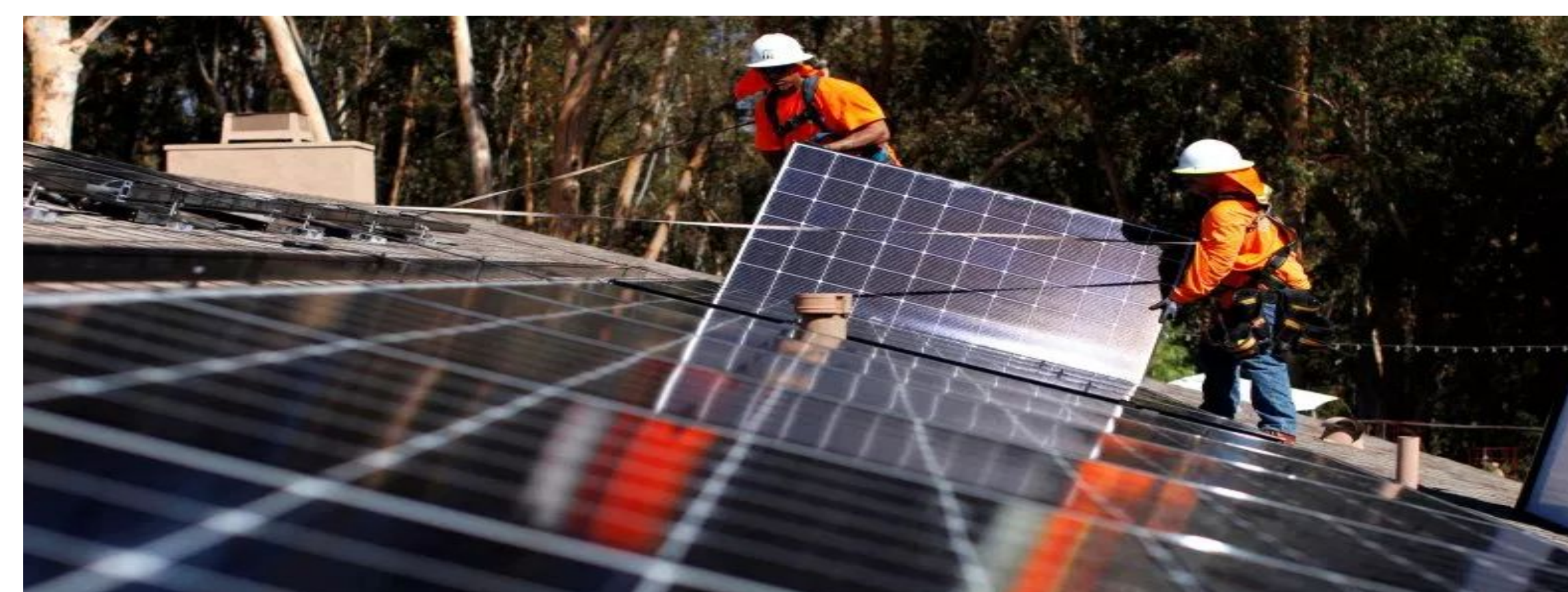
Installing solar panels on a home in Scripps Ranch, Calif. (Reuters photo: Mike Blake, 2017)
