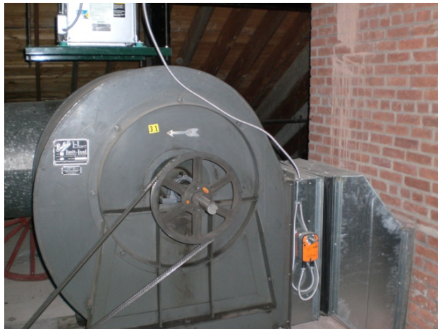
Figure 2.9 Secondary Ventilation System, Front View
