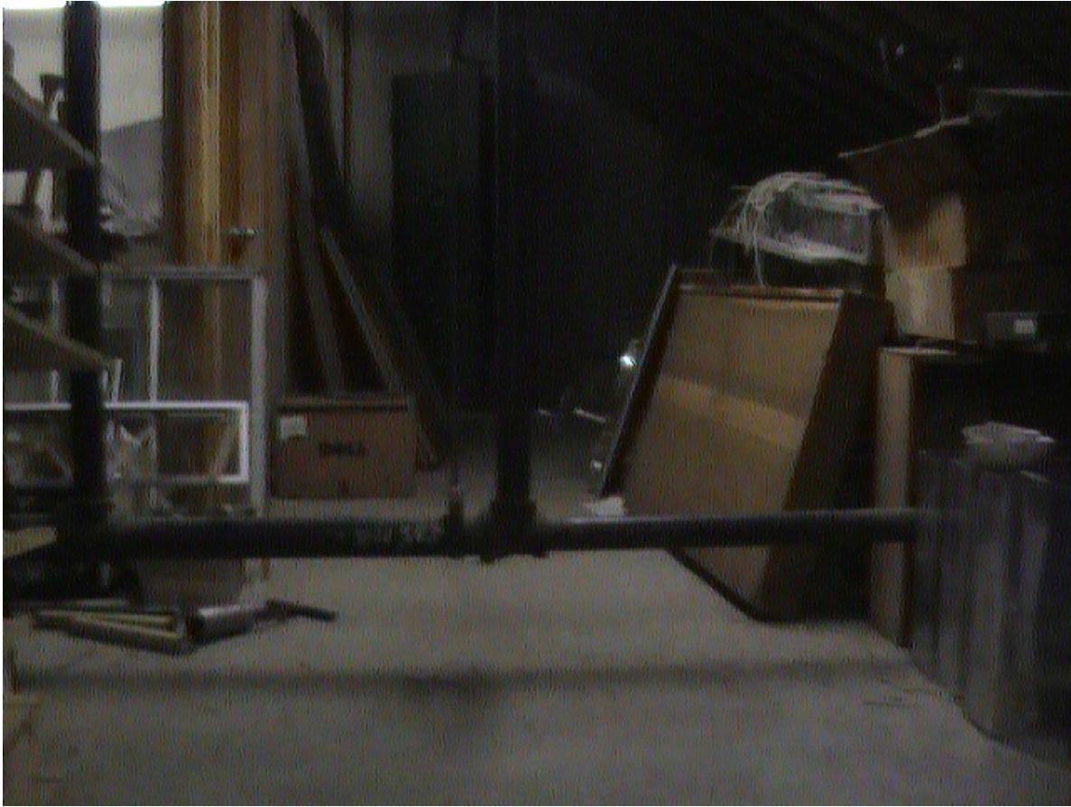
Figure 2.12 Problematic Sprinkler Pipe
