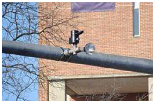
Figure 186: Traffic Preemption Device
