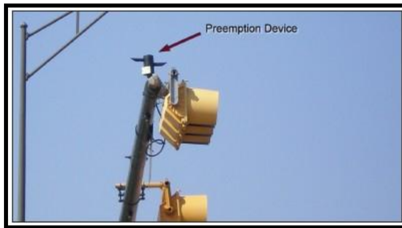
Figure 12: Traffic Preemption device installed on traffic light post
