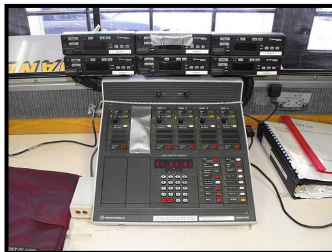
Figure 8: Motorola Centracom II console setup as a mobile dispatch setup
