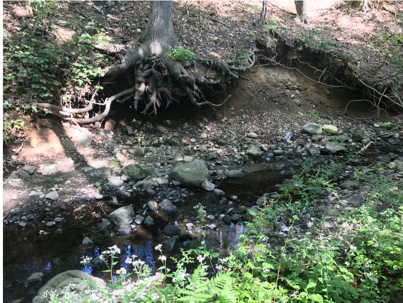
Figure 3: Erosion along Coal Mine Brook
