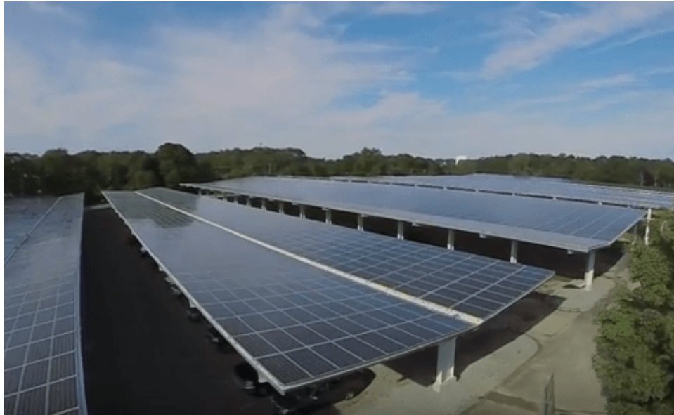
Figure 27: New England's Largest Solar Parking Canopy (SI Staff, 2015)
