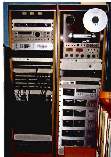
Fig. 2-4 Equipment Rack, Digital Recorders
