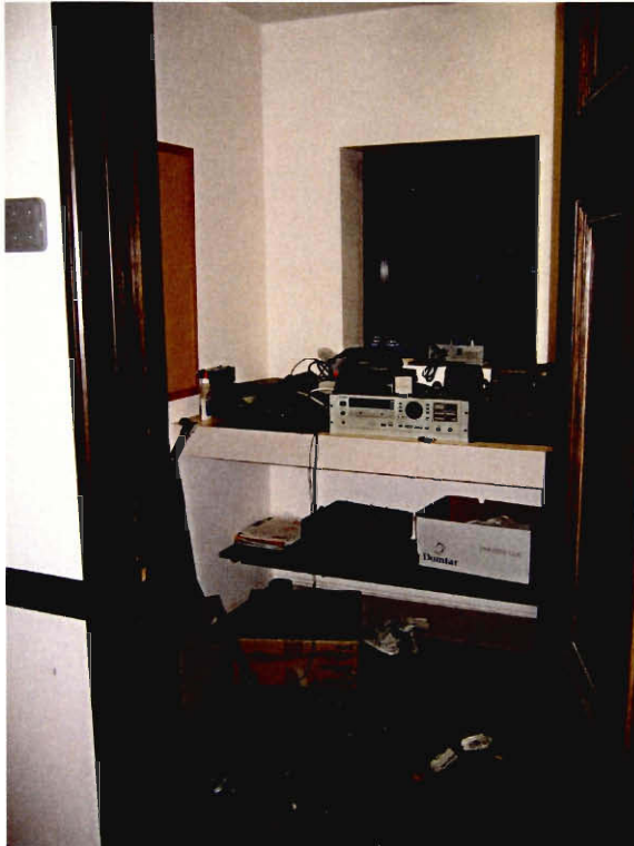
Fig. 3-16 Audio Closet Before Cleaning
