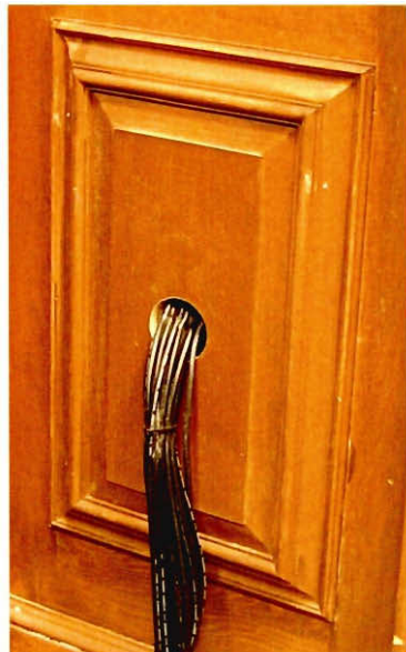
Fig. 3-38 Control Room Cabling Point of Entry
