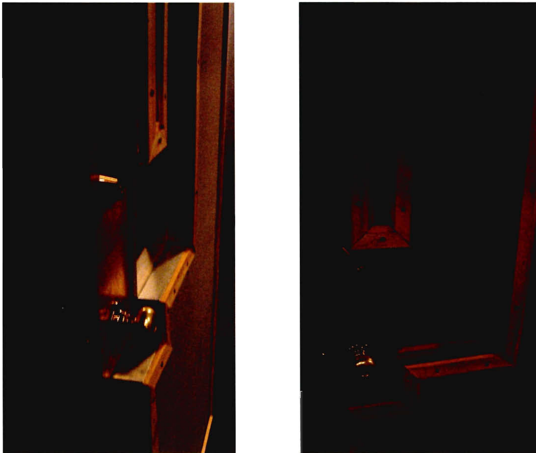
Fig. 2-13 Soundproof Doors Separating Environments
