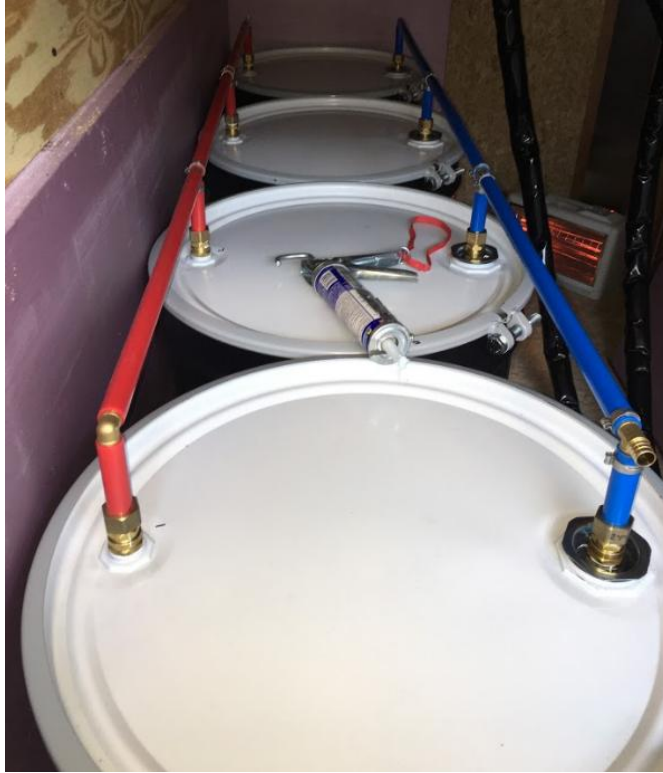
Figure 32: Line Piping Connecting Drums
