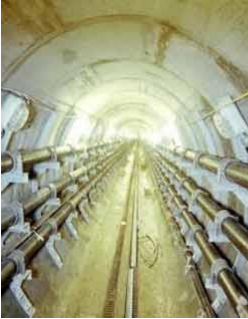
Figure 17: Cables within a tunnel (EMFS, 2014)
