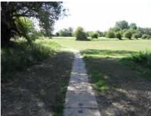
Figure 16: Cables Laid in a Trough Near Oxford (EMFS, 2014)
