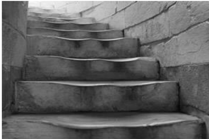
Figure 20 Worn Down Staircase
