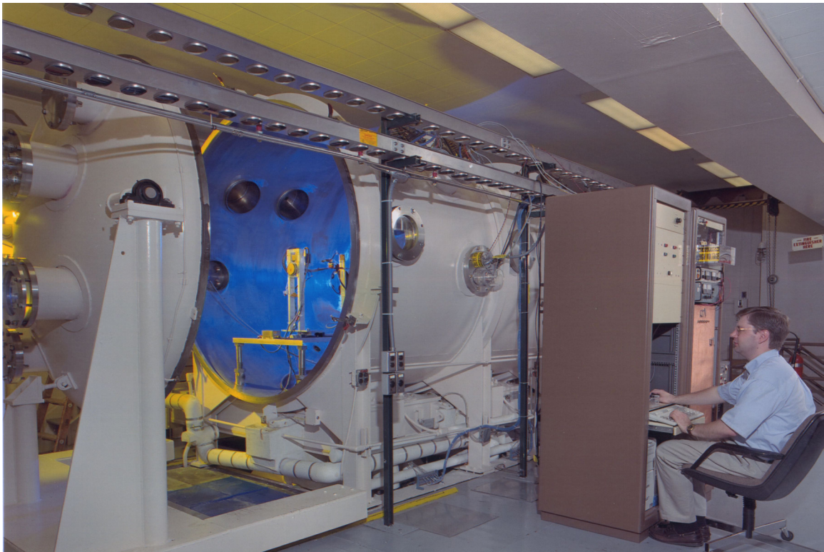
Figure 2.3 Vacuum facility and instrumentation racks.
