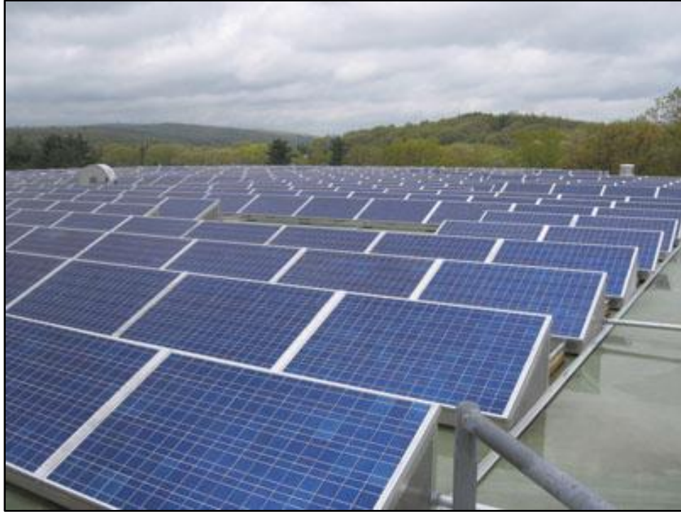
Figure 16: WSC Learning Resource Center PV array
