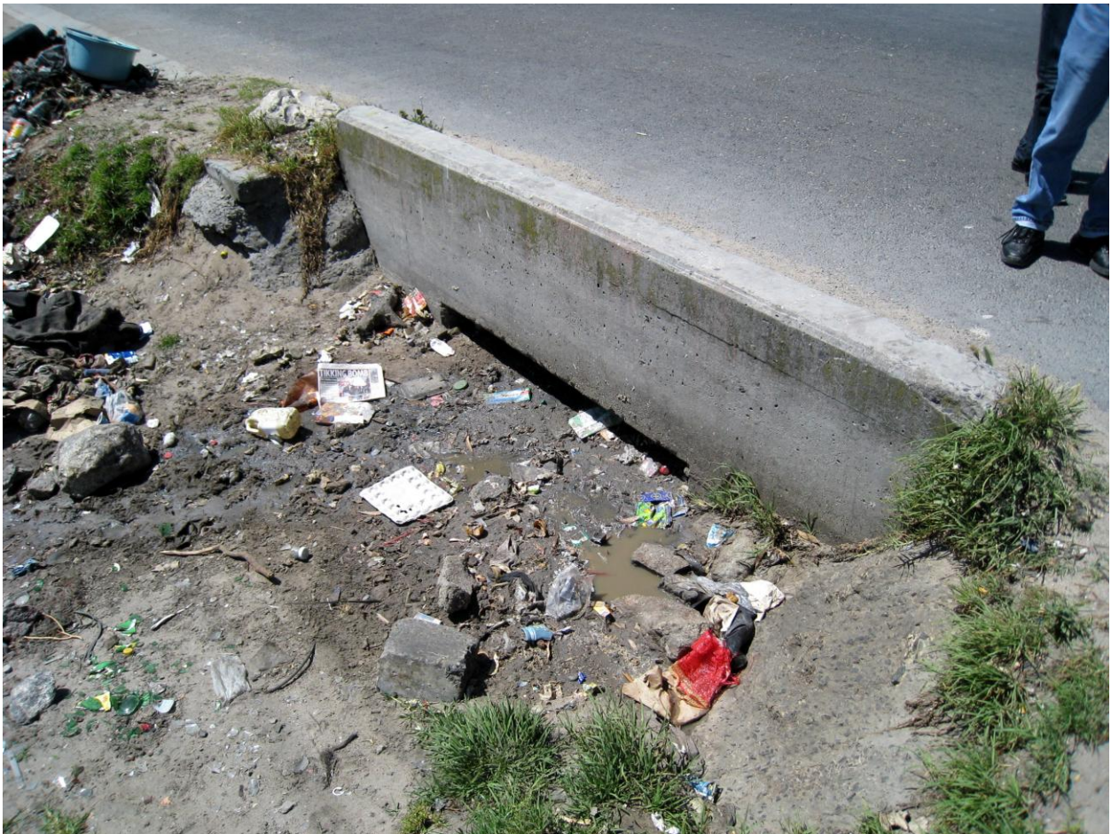
Figure 5: Silt and rubbish accumulation in drain
