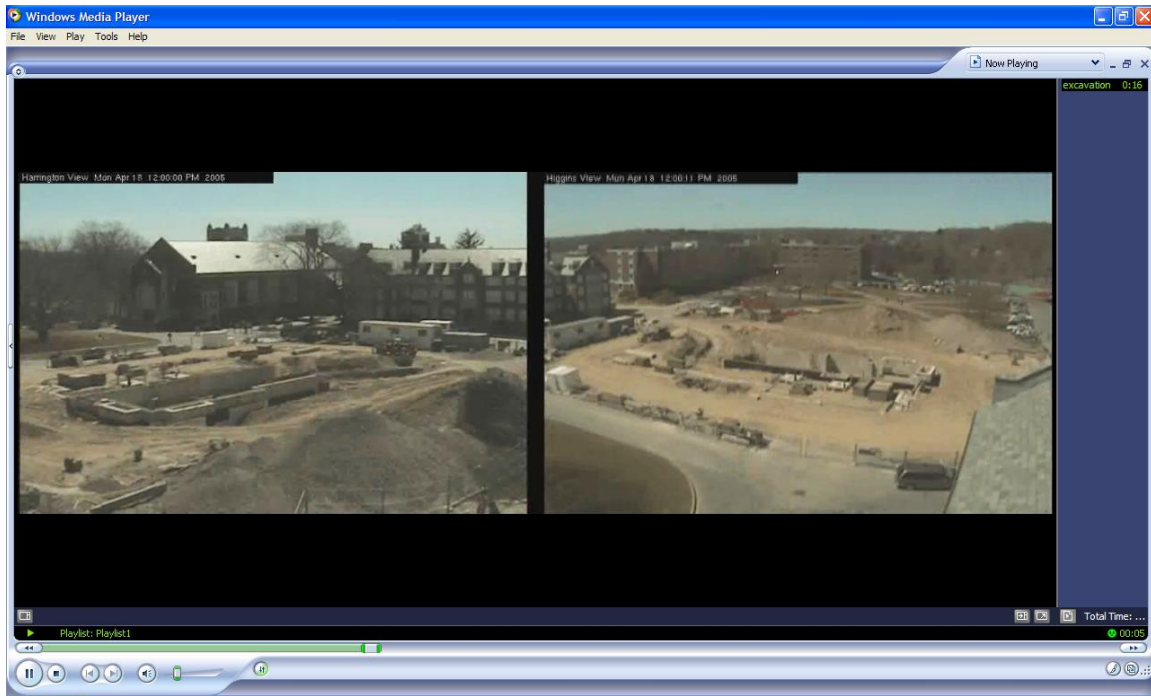
Figure 9 - Example of video footage provided from Higgins Labs (left) & Harrington Auditorium (right)
