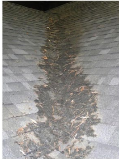
Figure 5: Damage to the roof covering after ignition of the pine needle debris in the valley 49 .
