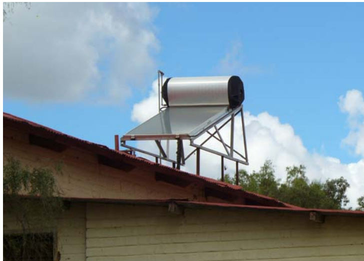
Figure 3 - Solar Water Heater
