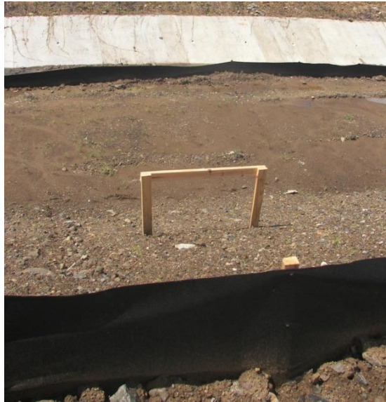
Figure 16 - Site 1 showing silt fences installed after soil erosion bridge (Photo Credit: Bryan Lee, 2011)
