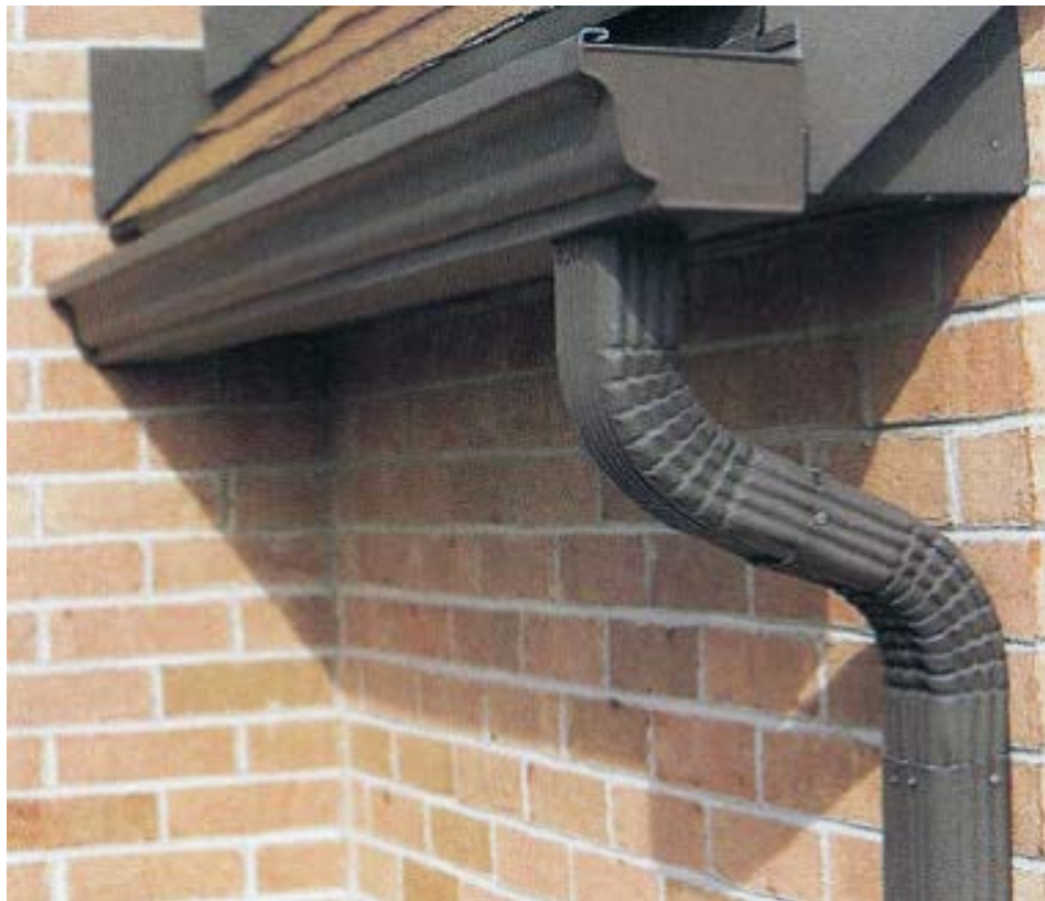
Figure 19: Elbow Connectors and Short Lengths of Downspout
