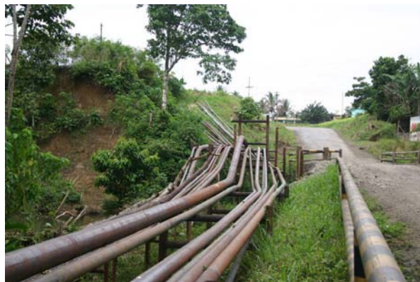
Figure 18: An example of the pipelines running through Ecuador (Doug Beltman, Stratus Consulting)
