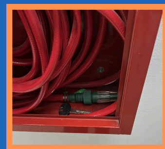
Photo 5: Key to the backyard hidden in firehose cabinet
