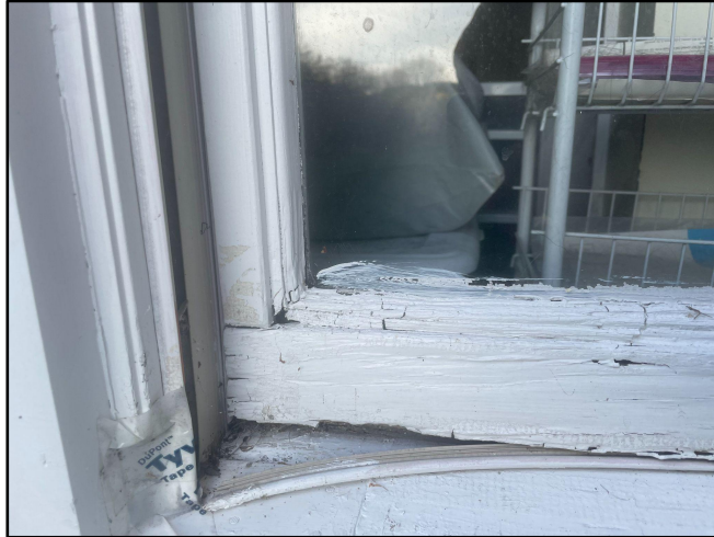
Figure 4.5 A deteriorated window is seen on the southern face of the basement-level facade at 42 Wolbach Road
